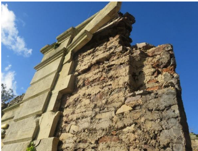
Photograph 3: A piece of ashlar which is hanging off the building.
