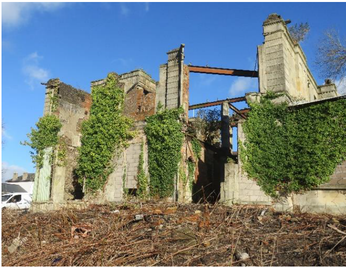
Photograph 2: Ivy growing up the walls of the building.
